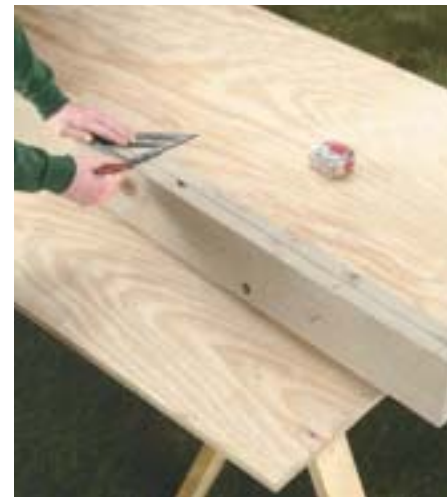
A. Tack together the rim joists, then mark the joist layout. Use a square to transfer the marks to the second rim joist.
