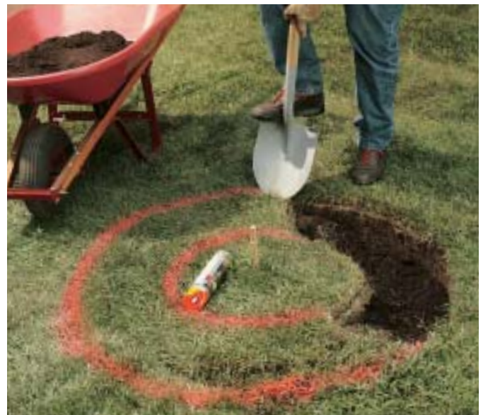
A. Outline the location of the footing using spray paint and a piece of string. Then dig a circular trench 10" deep.
