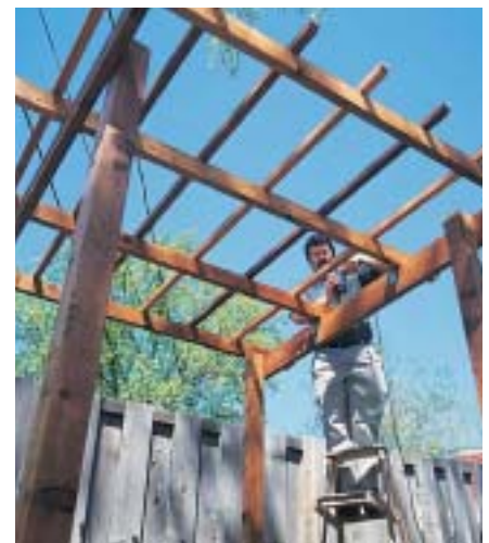
F. Space the cross strips 1 ft. apart and attach them to the rafters.
