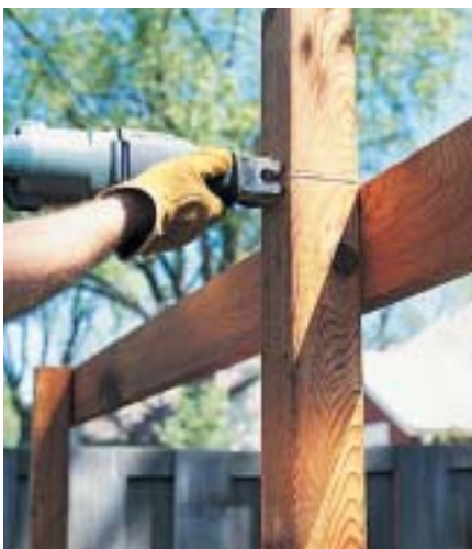
D. Attach the other tie beam and trim the tops of the posts flush with the tie beams.
