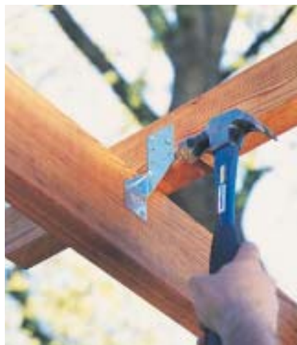
E. Attach the rafters to the tie beams with rafter ties and galvanized nails.
