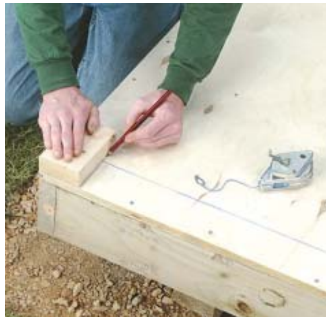
A. Use a block cut from plate material to lay out the bottom plates. Mark at the ends of each wall then snap a chalk line.
