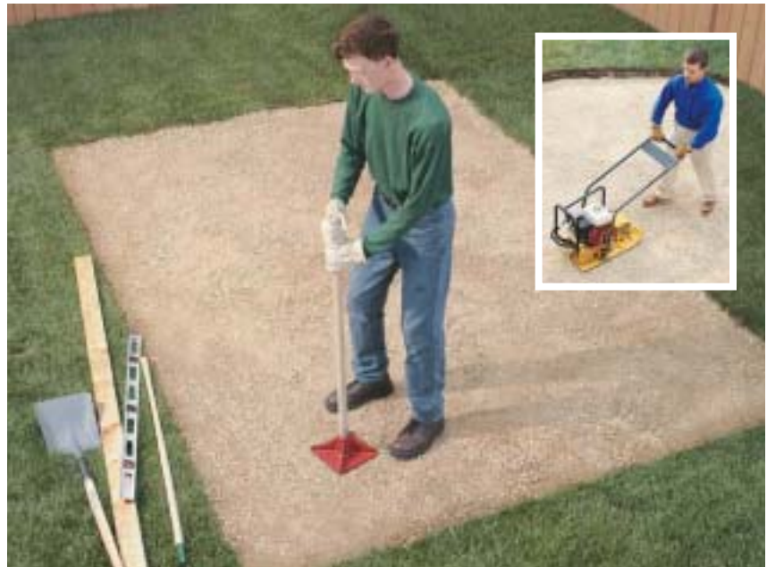
A. Excavate the building site and add a 4" layer of compactible gravel. Level, then tamp the gravel with a hand tamper or rented plate compactor (inset).
